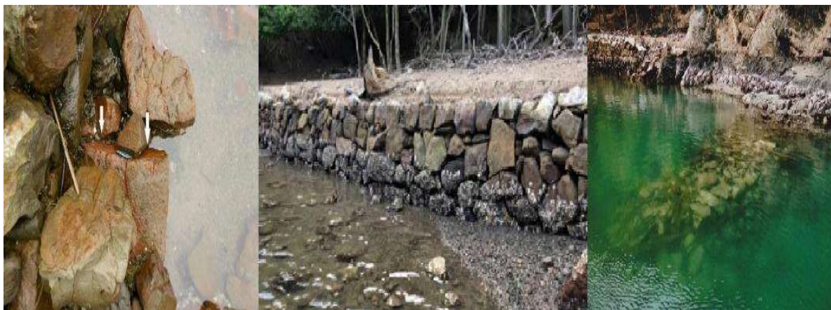
Figure 7: Iron Wedge on a Sandstone, Stone Masonry, and Submerged Jetty of Site D. (by M. Ooe)
