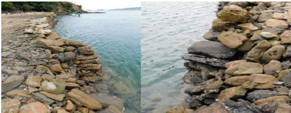
Figure 3: Collapsed Section of Site A. (by S. Yanagita)
